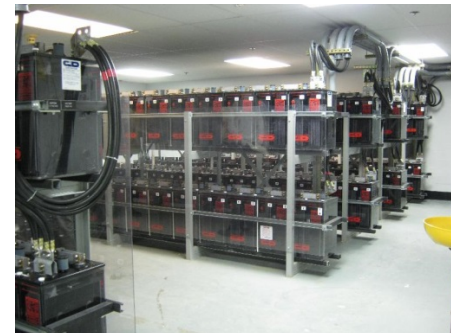
Building-scale battery array
