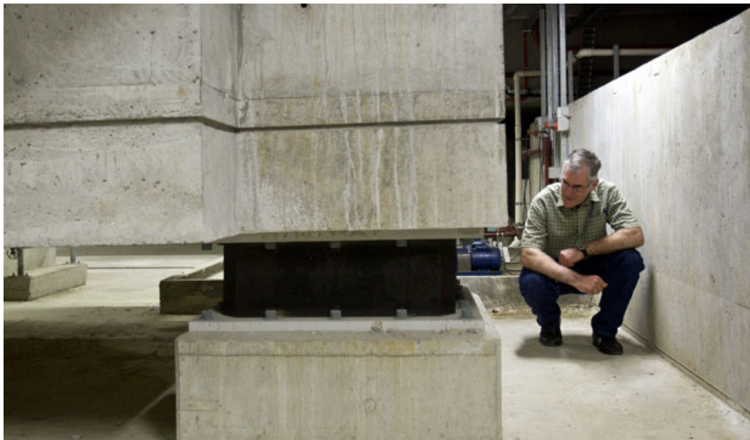
Figure 3. One of 45 seismic isolation bearings in the isolation galley of the Christchurch Women's Hospital, NZ, March 2013
