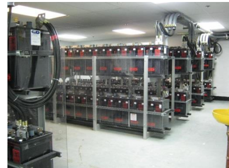
Building-scale battery array
